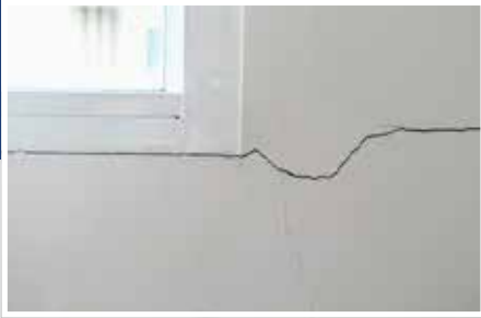
Interior Wall Cracks
