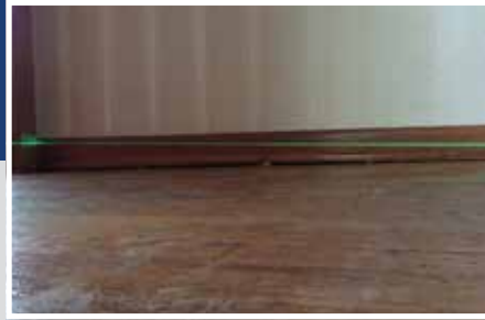
Separated Baseboards & Sagging Floors
