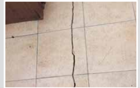
Cracks in Floors
