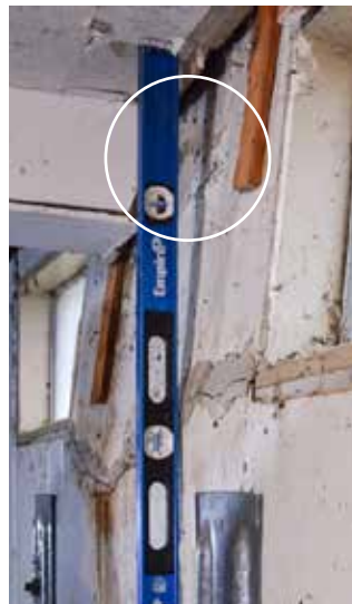
Wall is Severely Bowed in
