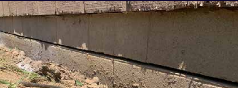
Before: Gap allowing moisture and pest intrusion.
