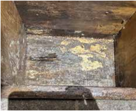
Wood rot in support columns and floor joists.
