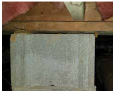
Bouncy floors can be caused by too much moisture in your crawl space.
